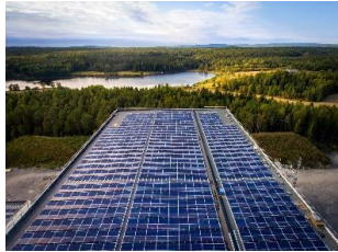
Asko and Unil: Owner's Engineer for a total of 12 MWp on C&I rooftops
