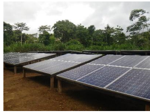
Cameroon: technical DD microgrid rural electrification
