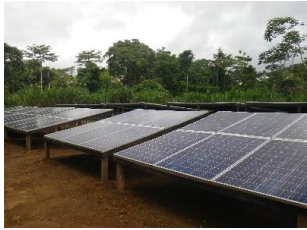
Cameroon: technical DD microgrid rural electrification
