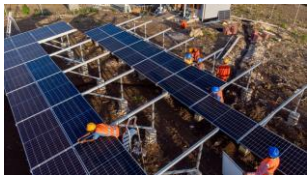
Zanzibar: design and procurement microgrid island power system
