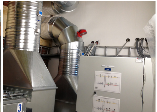
Top: New roof | Photo: Multiconsult Bottom: Ventilation, electro and automation | Photo: Multiconsult
